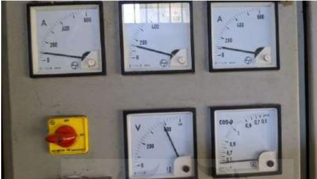
Meters Reading at MDB showing current and voltage of LV side
