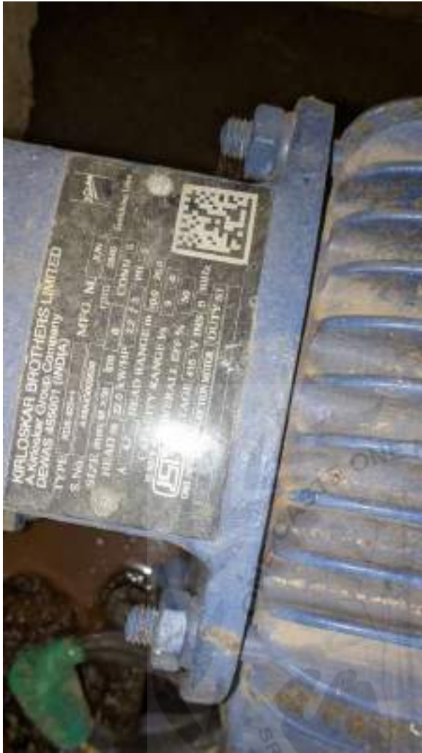
Name plate details of water pump set
