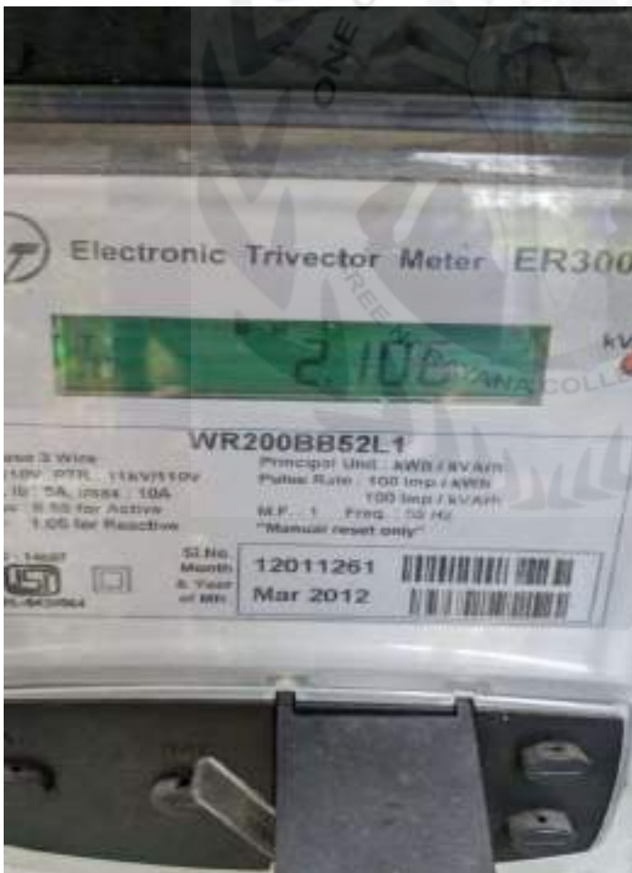
TOD metering at HV side showing current
